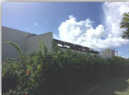
June 6, 2017 – Before encroachment was removed
